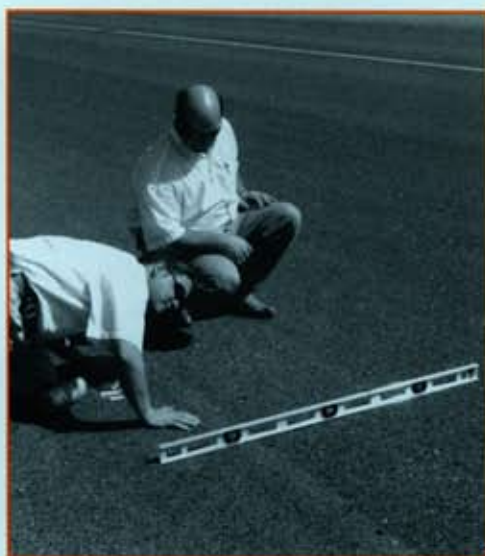
Matt Carden, APAC Tennessee, and Ronnie Goree, Asphalt Institute, try to find rutting on Taxiway N at Memphis Intl. Airport
